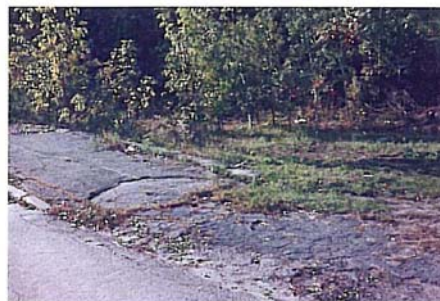
Deteriorated sidewalks do not provide an attractive facility for pedestrians
